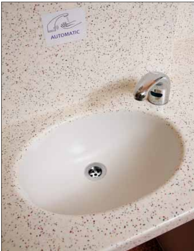
A separate wash-hand basin should be provided for use by staff conducting decontamination. This basin should be distinctly separate from the sinks used in decontamination
